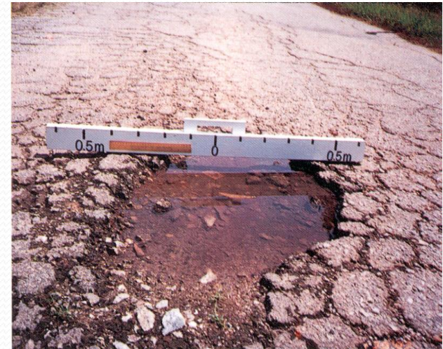
High Severity potholes with groups of potholes , depth >50\text{mm} and area >0.1\text{m}^2
