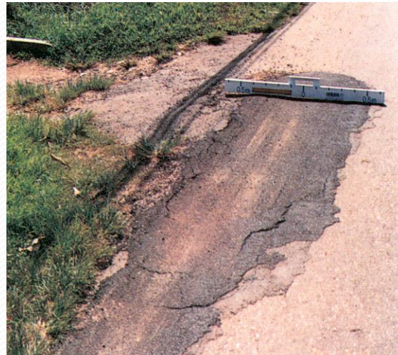
Patch with High Severity distress
