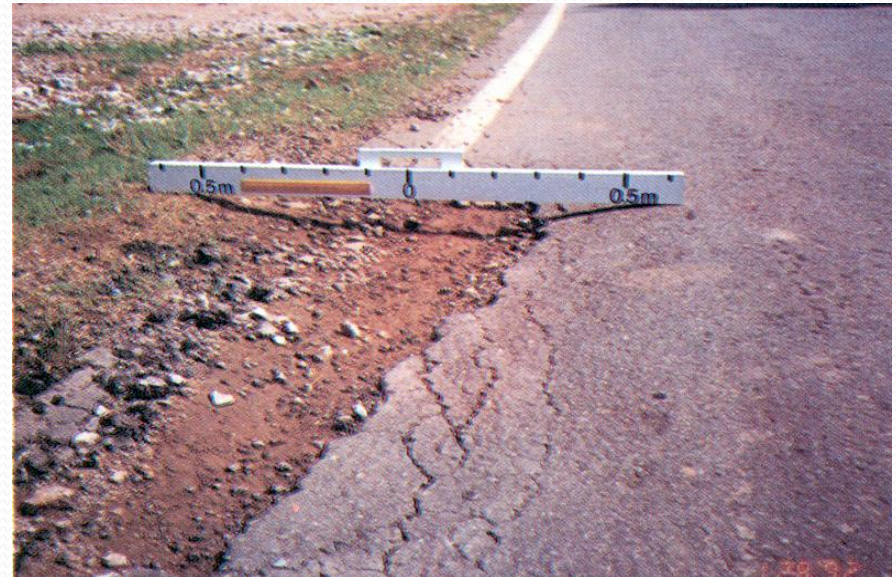
Severe Edge Break with considerable braek-ups
