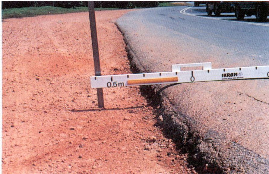
Severe Edge Drops-off height >100mm
