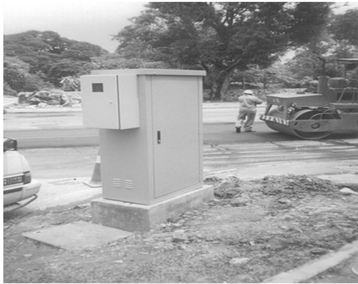
• Traffic Signal Controller and TNB Meter Panel
