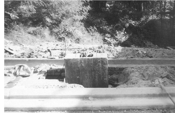
• Traffic Signal Controller Plinth
