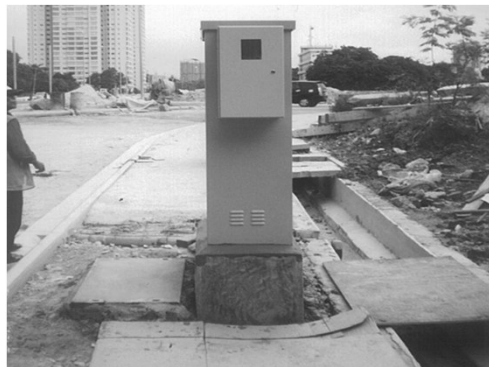
• Traffic Signal Controller and TNB Meter Panel
