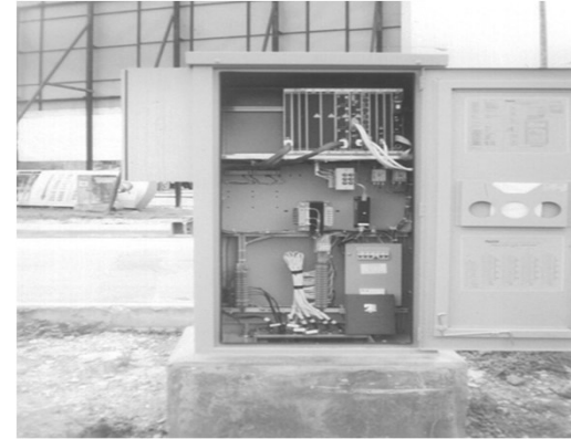
• Traffic Signal Controller and TNB Meter Panel
