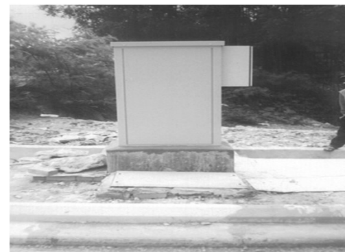
• Traffic Signal Controller and TNB Meter Panel
