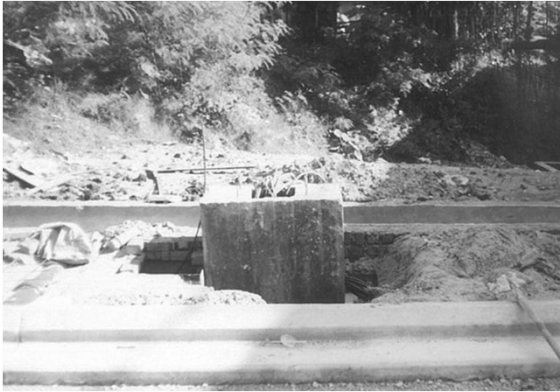
• Traffic Signal Controller Plinth
