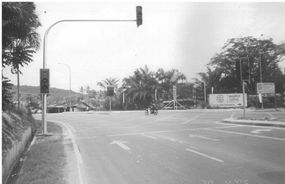
• Traffic Signal Overhead Pole (Mast Arm)
