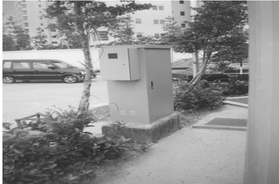
• Traffic Signal Controller and TNB Meter Panel
