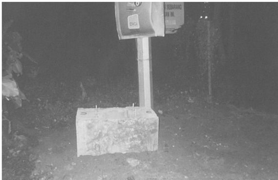
• Traffic Signal Controller Plinth
