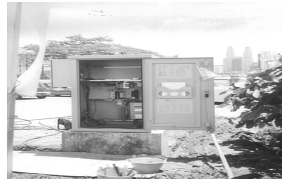
• Traffic Signal Controller and TNB Meter Panel
