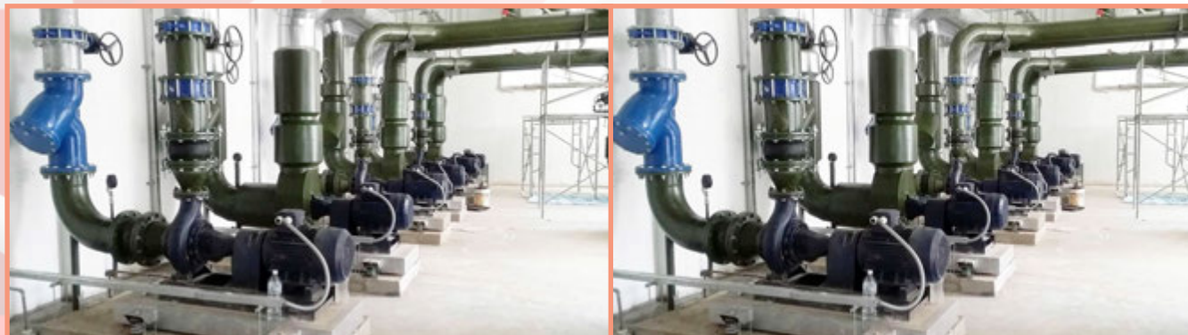
Peralatan Water Cooled Chiller Dan Pam Di Chiller Plant
