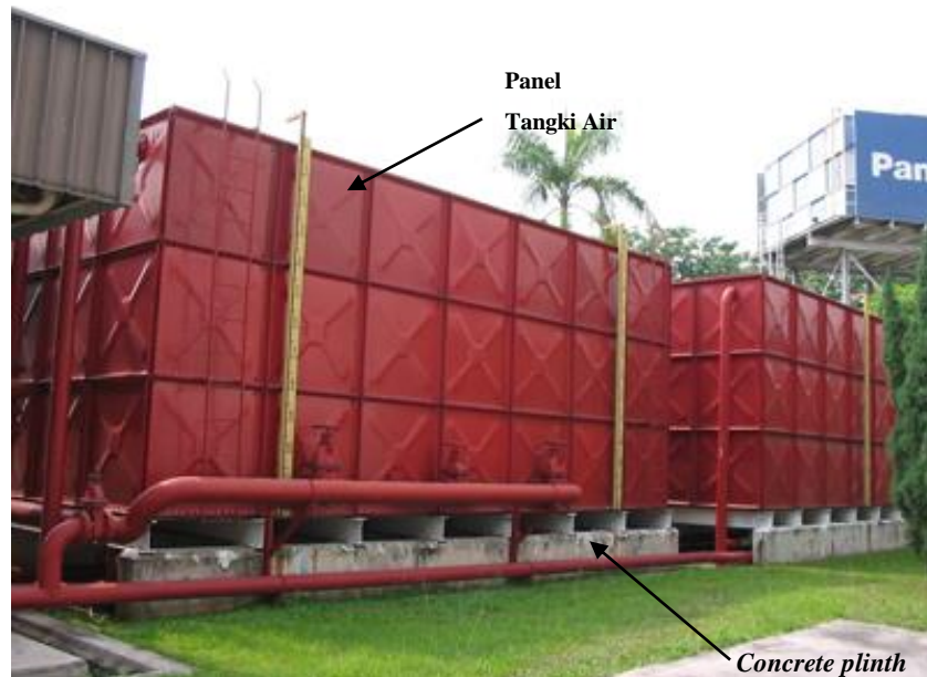
GAMBAR 1.1: CONTOH TANGKI SIMPANAN AIR JENIS PRESSED STEEL HOT DIPPED GALVANIZED .
