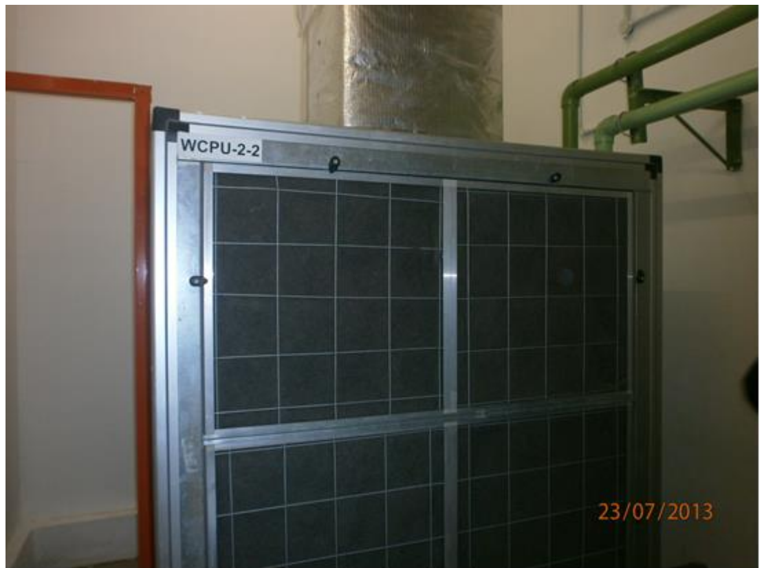
Figure 4.1 Picture of Current Air Handling Unit at level 2. Using VRF the AHUs will no longer be used.
