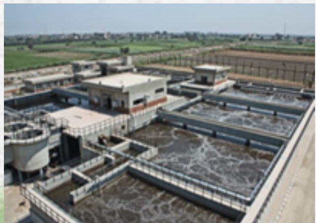
Figure 4: Sequence Batch Reactor Plant
