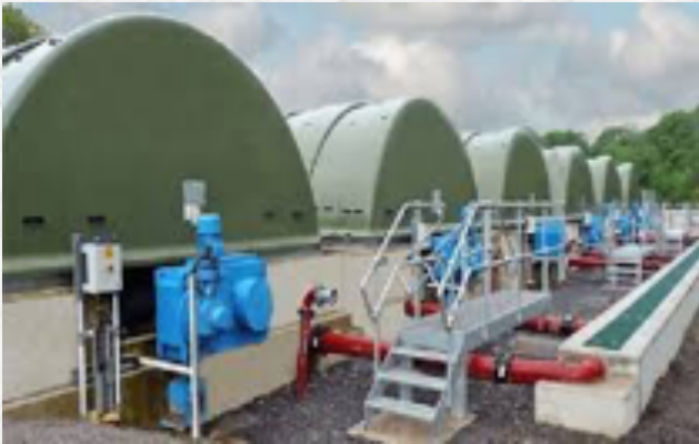
Figure 1: Rotating Biological Contactor
