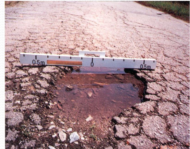
High Severity potholes with groups of potholes , depth >50mm and area >0.1m 2
