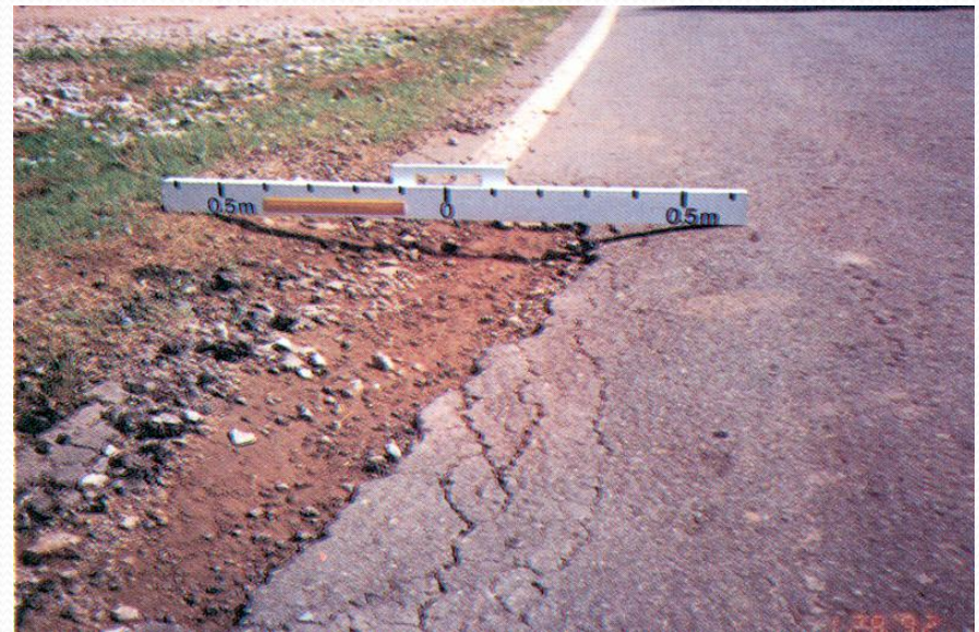
Severe Edge Break with considerable braek-ups
