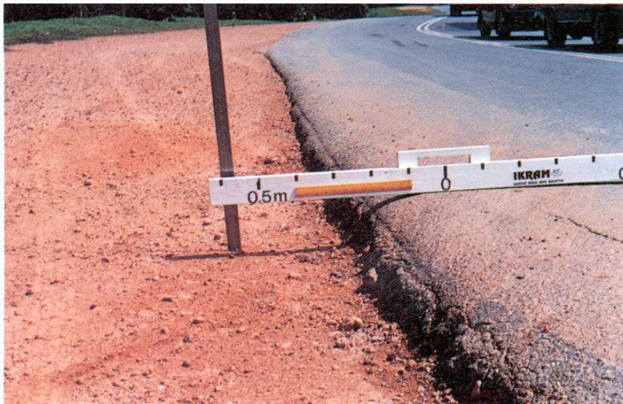
Severe Edge Drops-off height >100mm
