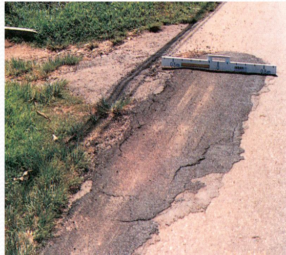
Patch with High Severity distress
