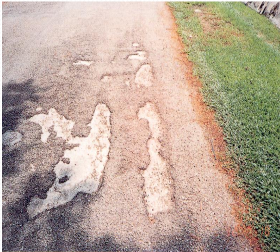
High Severity delamination with a group of delaminations
