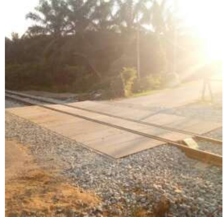
Inspection work by JKR & contractor to check on defect and settlement on the level crossing
