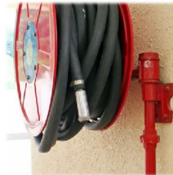
Hose Reel System
