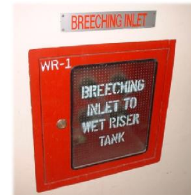
Wet Riser System
