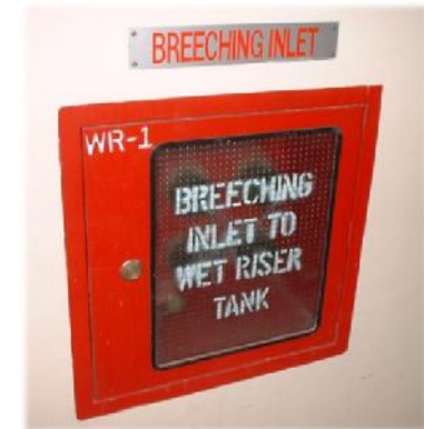
Wet Riser System
