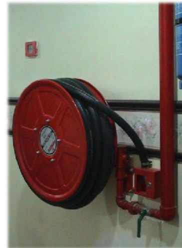
Hose Reel System
