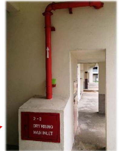
Dry Riser System
