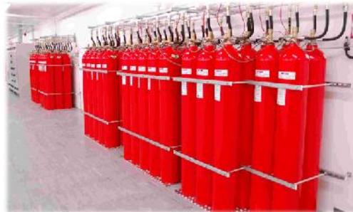
Fire Suppression Extinguishing System
