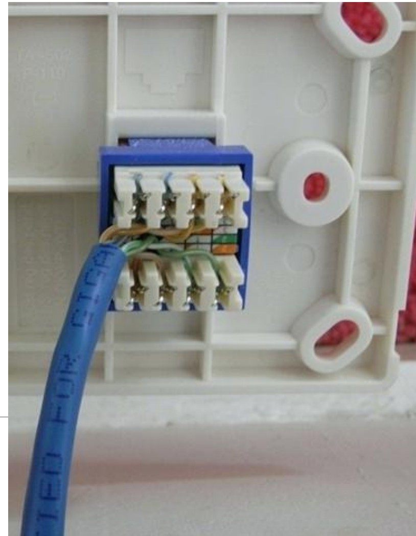
Faceplate with RJ 45 modular jack (termination of UTP Cat.6 cable at the User side)
