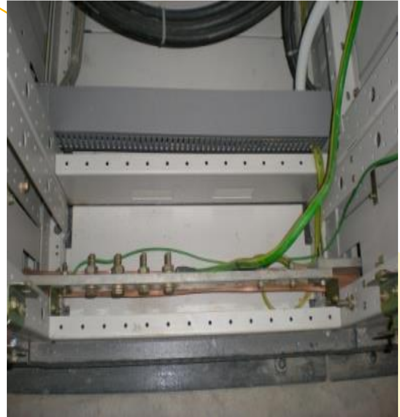
Main Earthing Bar
