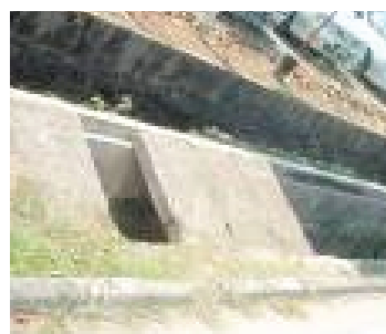
Precast concrete slab hilang/pecah.
