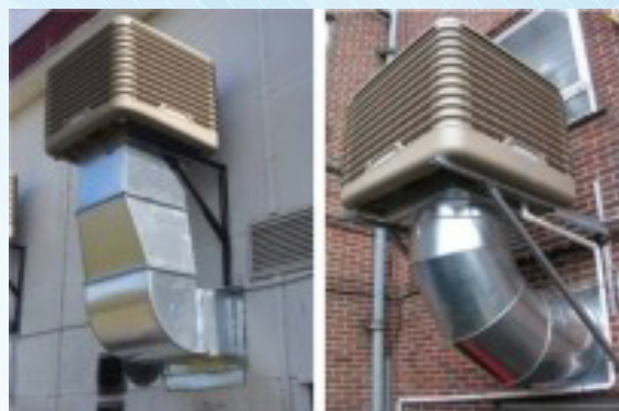
Figure 2. Evaporative cooling installed at site ( http://www.ecocooling.co.uk/products/install.php , accessed on 10/05/2017).
