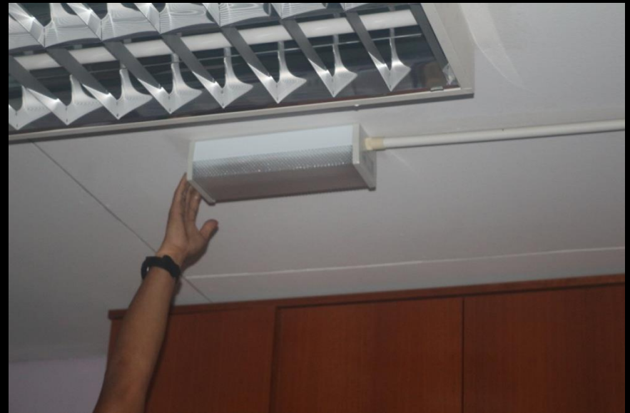
KEROSAKAN 'EMERGENCY LIGHT'
