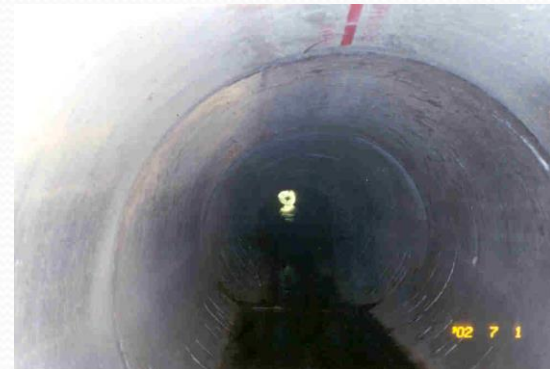
Surface undulations on the inside of culvert
