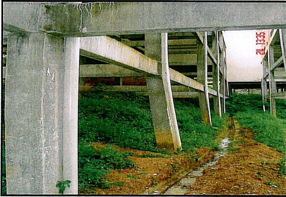
Plate 1C : Columns deflected towards the lake side and drainage facilities heavily silted
