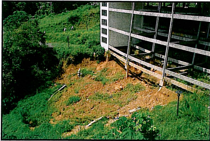
Plate 1A : Slip at the edge and below the building
