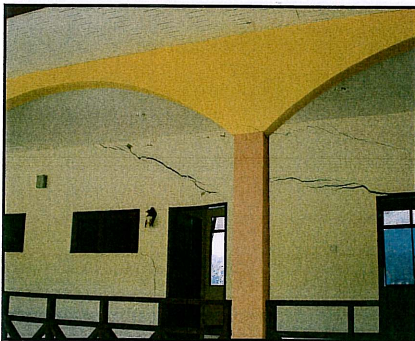
Plate 1B : Hairline cracks in localized beams and walls
