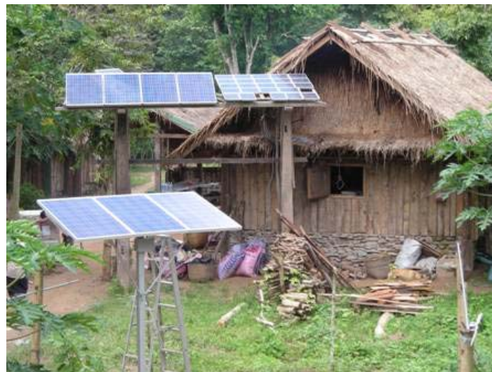
Solar Home System in Laos (Source: www.unep.org )
