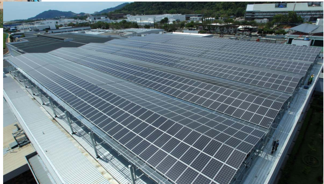
646 kWp, Robert Bosch (M) Sdn Bhd, Penang
