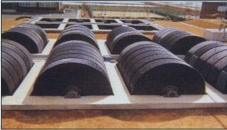
Rotating Biological Contactor (RBC)
