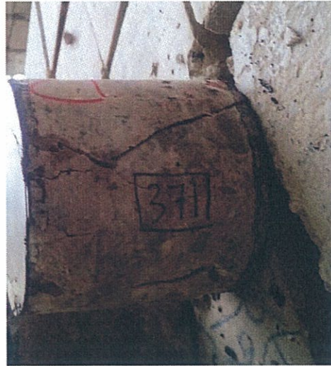
The crushed Concrete Core extracted from Pier 5.
