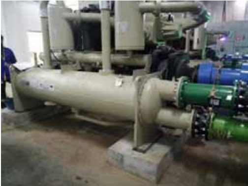
Unit Chiller Jenis Variable Speed Drive (VSD) Water Cooled Screw berkapasiti 250 RT di Chiller Plant Room
