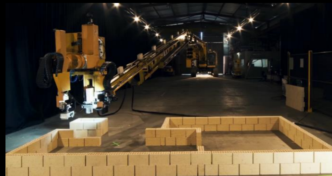
The grant brick laying robot can build entire house in just two days.
