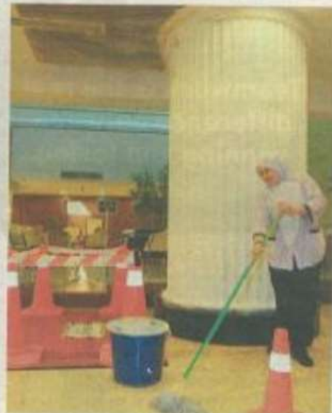
A worker cleans a pillar caused by a leak in the roof of Parliament House yesterday. — NST picture by Ishari Ariffin
