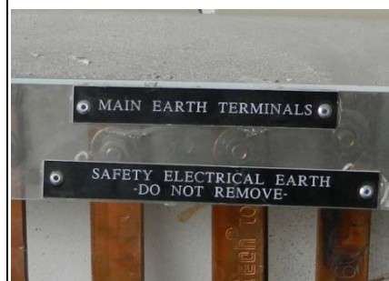
Permanent label 'Main Earthing Bar - Safety Electrical Connections - Do Not Remove'
