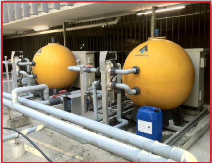
Sistem Non Chemical Condensate Water Treatment ▲
