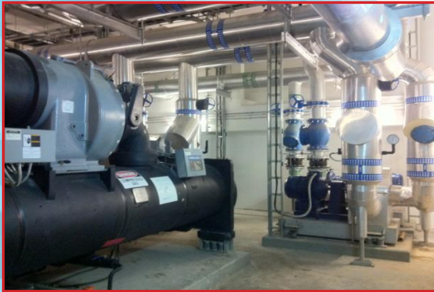
▲ High Efficiency Water Cooled Chiller
