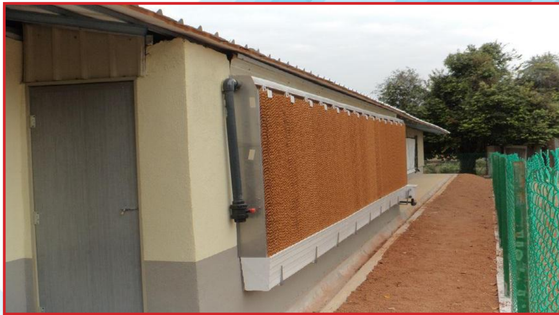
◀ Cooling pad (Water cool system)
