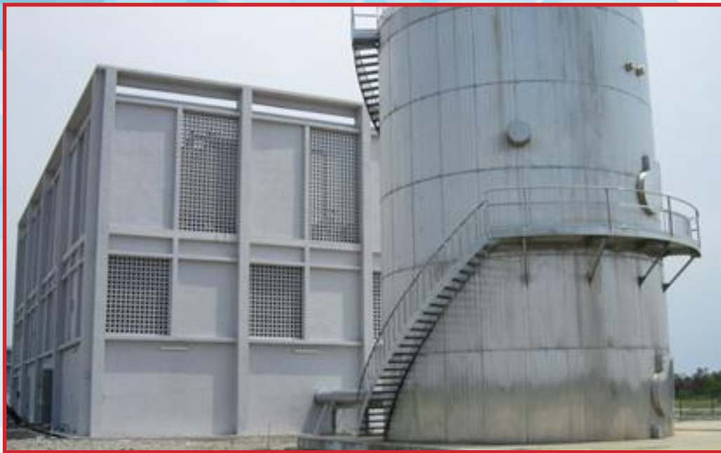
▲ M&E Plant Room
