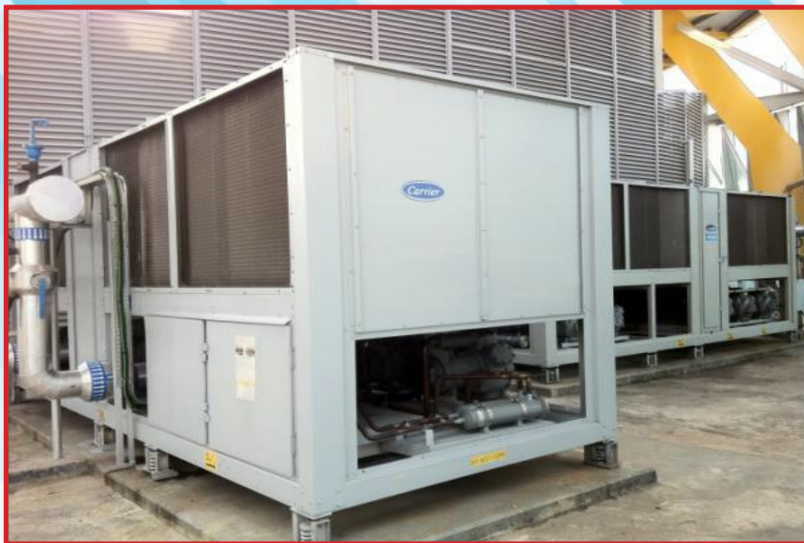
▲ Air Cooled Chiller
