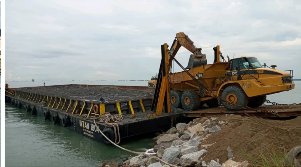
At temporary jetty, barge is unloaded. Excavator load dredge material into articulated dump truck
