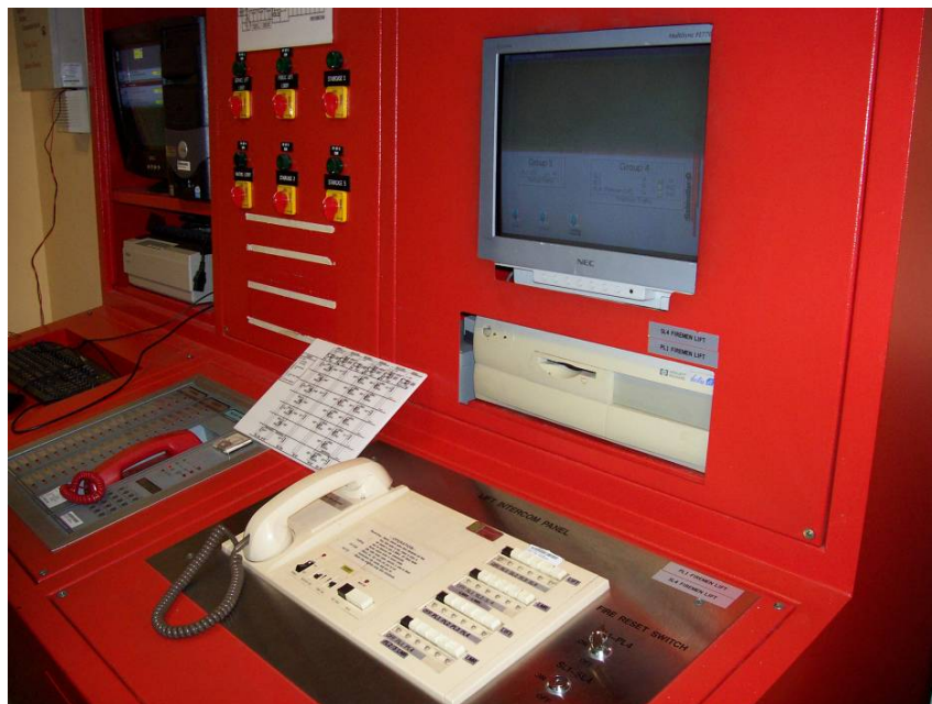
Gambar 2 : Main Fire Alarm Panel ( Di Bilik Kawalan Ground Floor )
