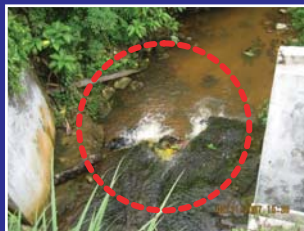
Under scour to apron slab at outlet.
