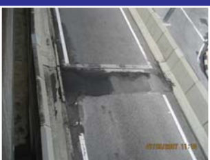
Adjacent pavement to compression seal joint detached.
