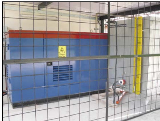
Figure 3.8 : 21.6 kW diesel generator at SK Penontomon (Source : Abdul Muhaimin Mahmud)
