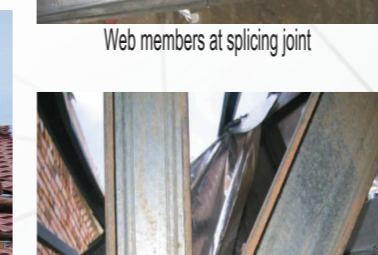
Wrongly drilled holes on the bottom chord of a truss
