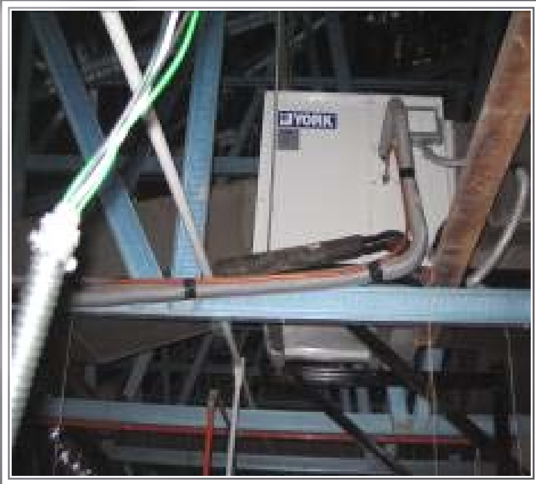
AHU tanpa secondary drain pan
