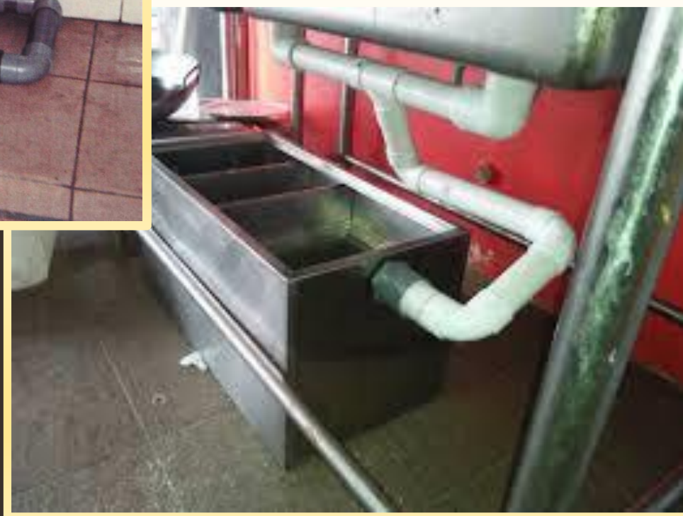
Grease trap (kitchen)
