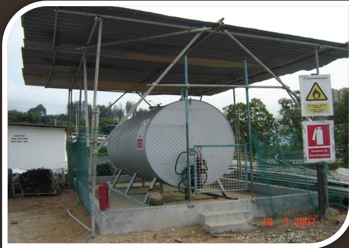
Containment Bund for Skid Tank
