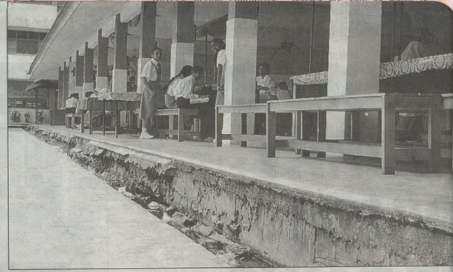
CAVING IN: The back part of the assembly area that has sunk
