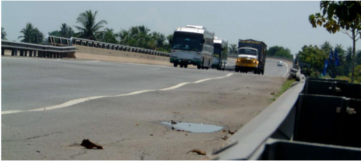
Fig. 7. 'Mushrooms' and undulating surface on expressway.
