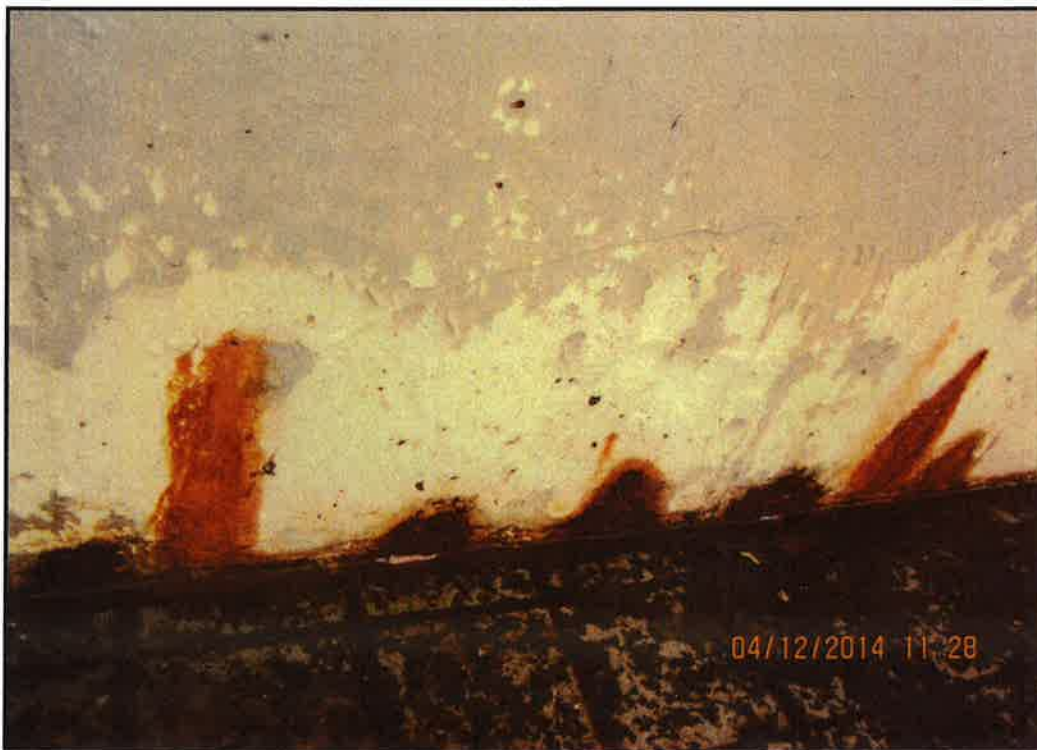
Gambar 17: Kesan pengaratan besi parapet wall
