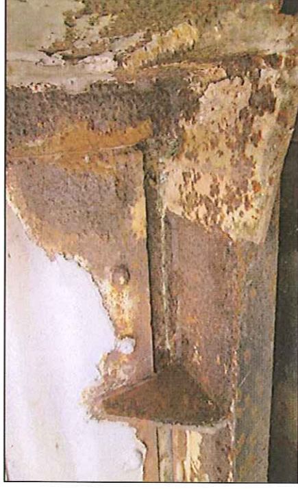
Picture M – S6 – P19 and M – S6 – P20 Moderate corrosion on steel plate.
