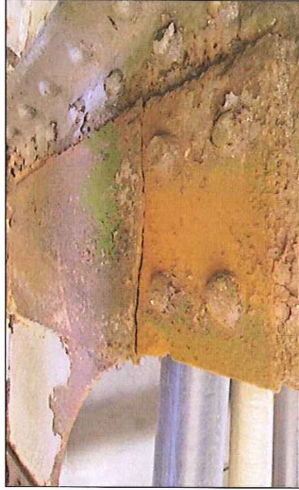
Picture M – S6 – P17 and M – S6 – P18 Moderate corrosion and crack line on steel plate near expansion joint.
