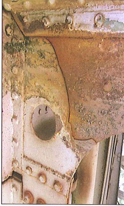
Picture M – S5 – P19 and M – S5 – P20 Moderate corrosion and crack line on steel plate.
