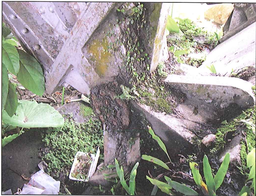
Picture B3 & B4 :- Some of the bridge's steel bearings with debris/vegetation accumulation and minor rusting. General maintenance works to remove all such vegetation growth with cleaning of the minor rust and re-greasing have been recommended.
