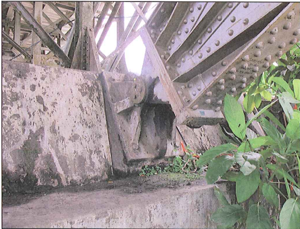
Picture B1 & B2 :- The bridge's steel bearings were found to be generally in good operating condition. General maintenance works for cleaning and re-greasing have been recommended.
