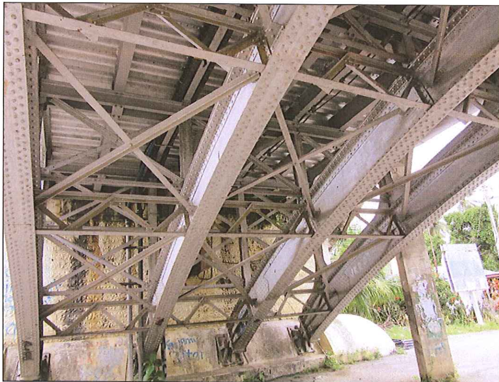
Picture 7 & 8 : General views of the bridge's soffit at the North-West end span.
