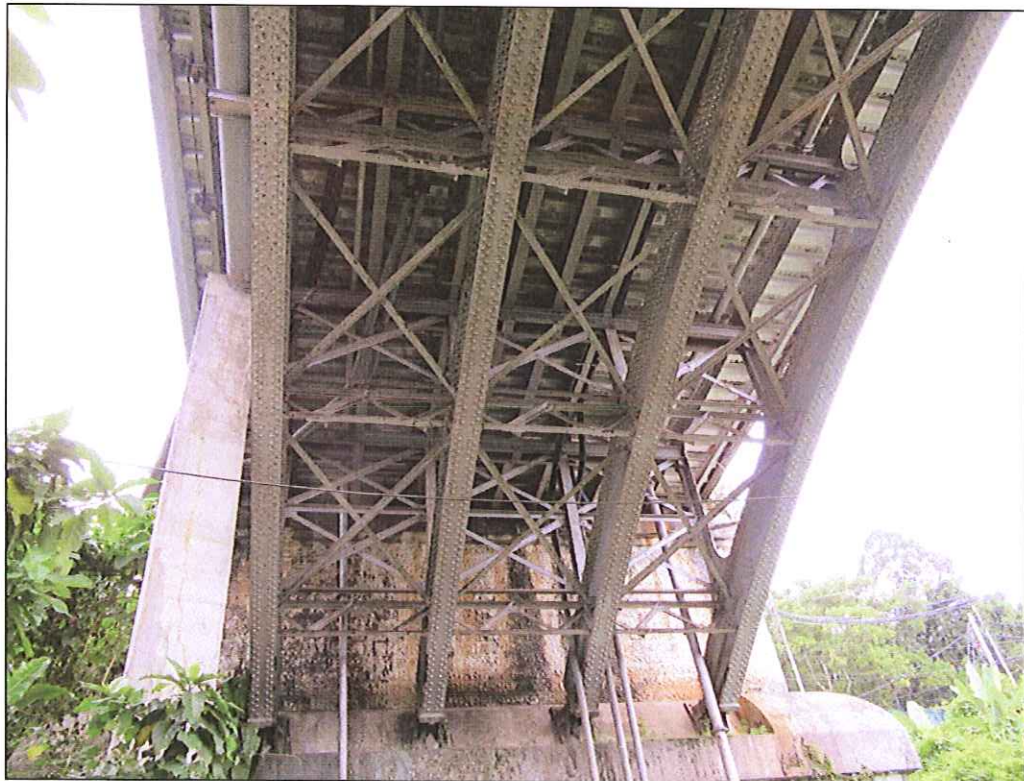
Picture 9 & 10 : General views of the bridge's soffit at the South-East end span.
