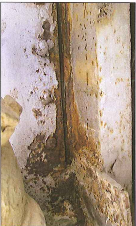
Picture M – S3 – P33 and M – S3 – P34 Moderate corrosion on steel frame.
