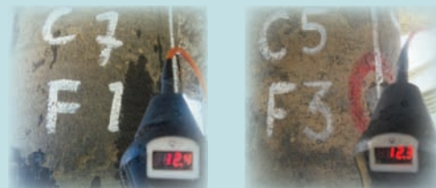
Gambar 5 & 6: Ultrasonic Thickness Test
