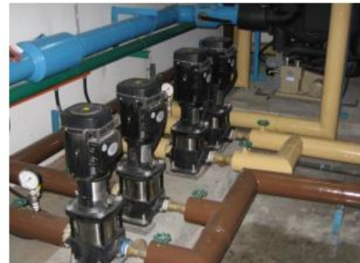
*Hot water Pump
