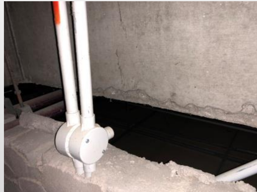
Dinding bukan full height
