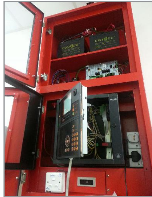
Fire Alarm Panel
