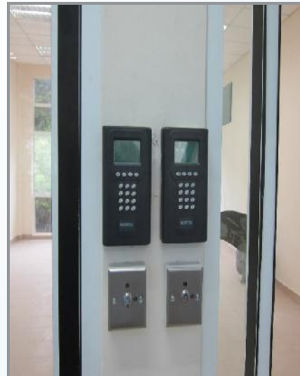
Sistem Integrated Building Management & Security System (IBMS)
