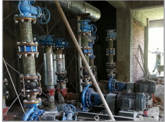
Chilled Water Pump
