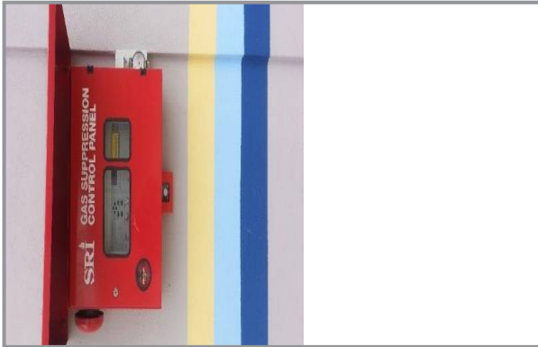
Clean Agent Control Panel
