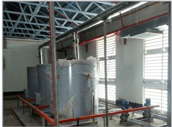
Hot water calorifier dan circulating pump
