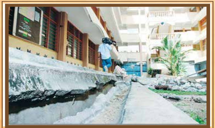
Figure 4: Road Settlement at Sekolah Menengah Kebangsaan (SMK) Setapak Indah
