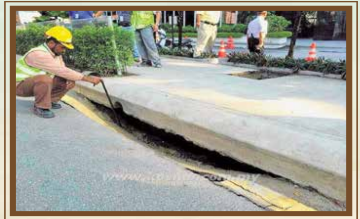
Figure 2: Road Settlement at Jalan Bukit Bintang
