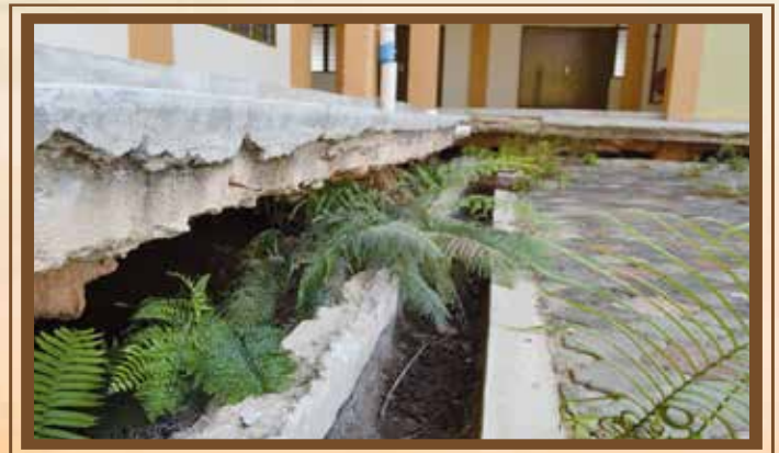
Figure 3: Building Settlement at Sekolah Menengah Kebangsaan (SMK) Alor Limbat
