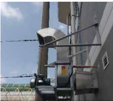
Kitchen hood Dilengkapi Sistem Wet Chemical Fire Suppression
