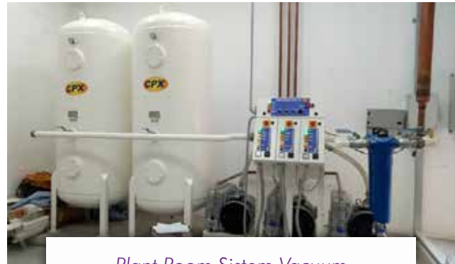
Plant Room Sistem Vacuum
