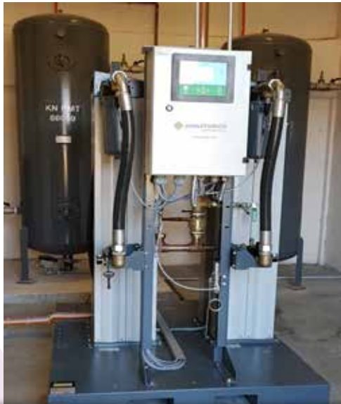
Plant Room Sistem Compressor (MA4)
