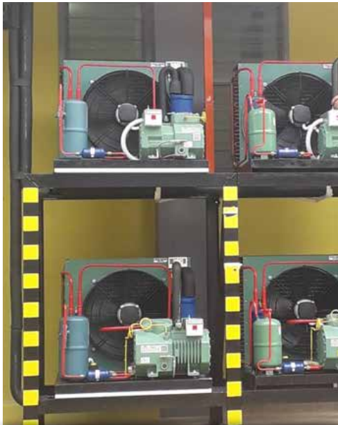
Condensing Unit Bagi Freezer
