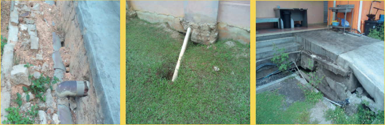
Figure 1: Damage to the existing drainage system due to soil settlement at Politeknik Sultan Idris Shah, Sabak Bernam, Selangor.
