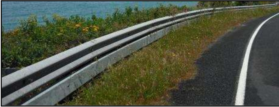
Figure 8.2: Photograph of Rub Rail Fitted To an Existing W-Beam (Source: Safe Direction)
