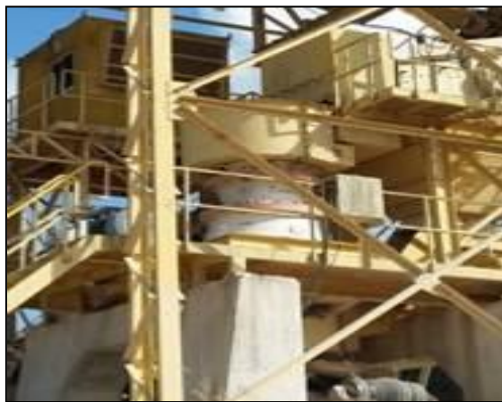
Rajah 3.1.2.1 : Loji Secondary Crusher
