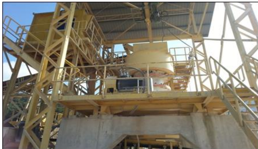
Rajah 4.5.3.1 : Loji Secondary Crusher
