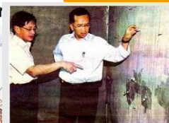
Leaky RM18m aquatic centre shut down
