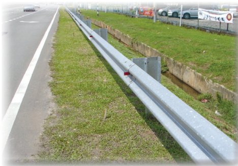
Guardrail TL-2, jarak tiang asas 4 meter.
