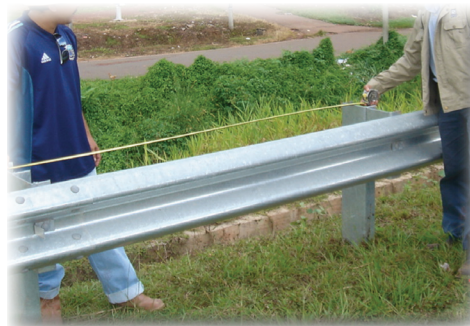
Guardrail TL-3, jarak tiang asas 2 meter.
