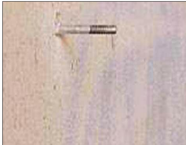
Figure 15.5.3: Exposed probe embedded in concrete structure.
