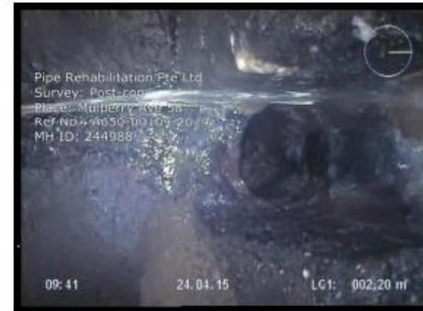
Photo: 244988-042415-M10.JPG General photograph, incoming pipe 1
