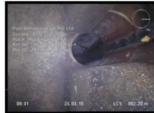
Photo: 244988-042415-M11.JPG General photograph, incoming pipe 2
