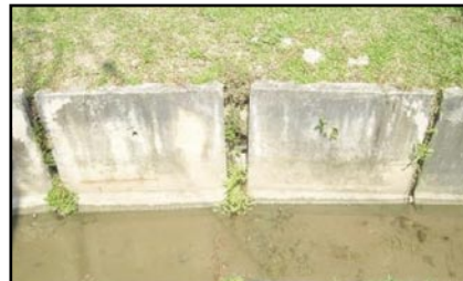
GAMBAR 4 : GAP ANTARA JOINT > 6mm
