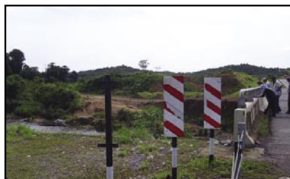
GAMBAR 8 : VERTICAL BRIDGE PANEL HILANG/ROSAK
