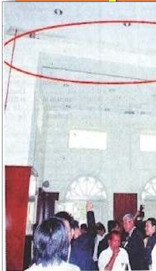
The original spot of the cornice that fell (circled) at the top of the state assembly building. (Inset) Tan Cheng Liang (centre) taking a closer look at the fallen cornice.
