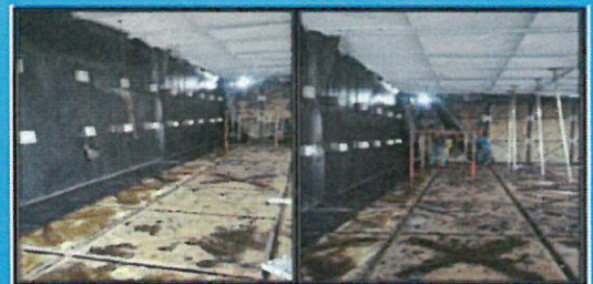
PRESSED STEEL TANK HDPE LINING
